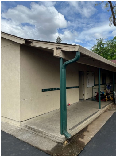
Dry rotted beam - before
